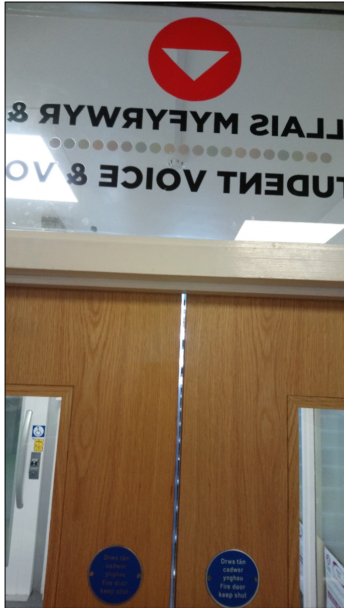
Figure 5 – Excessive gap between door leaves
